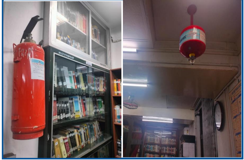
Fire Extinguishing System
